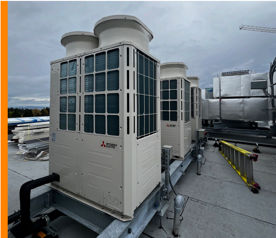
Mitsubishi City Multi air source heat pump (Photo credit: Introba)
