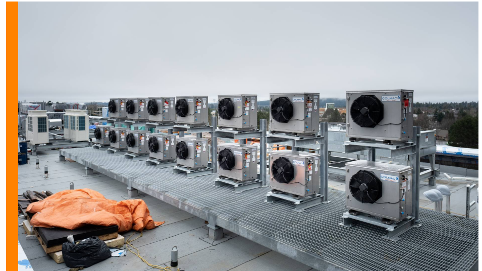
Colmac air source heat pumps for domestic hot water (Photo credit: Perkins+Will Architects)
