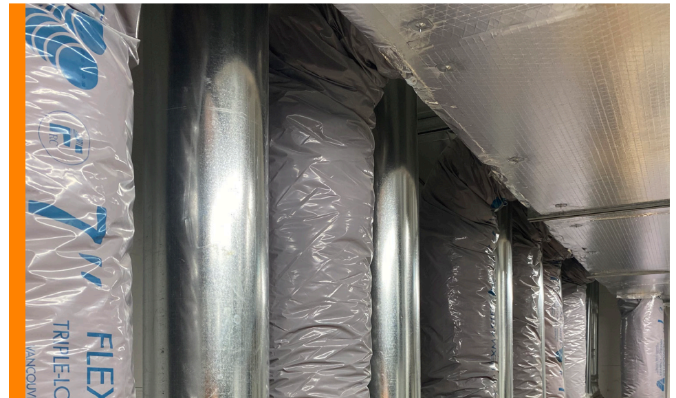
Supply (insulated) and return ventilation ducting.
