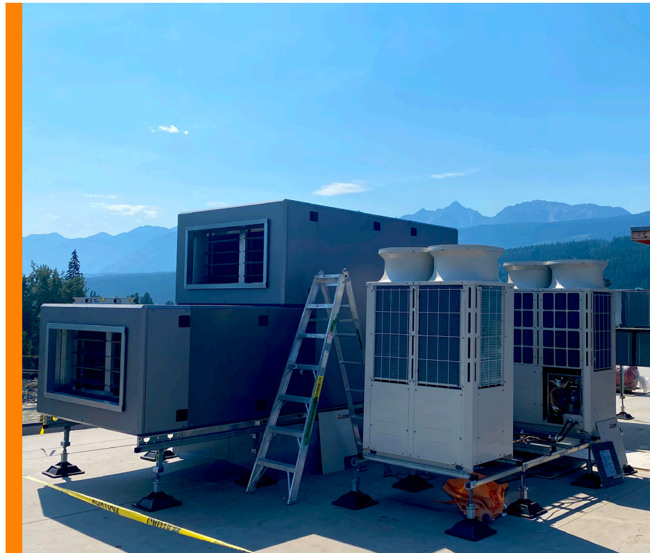
Swegon energy recovery ventilator connected to Mitsubishi heat pumps.
