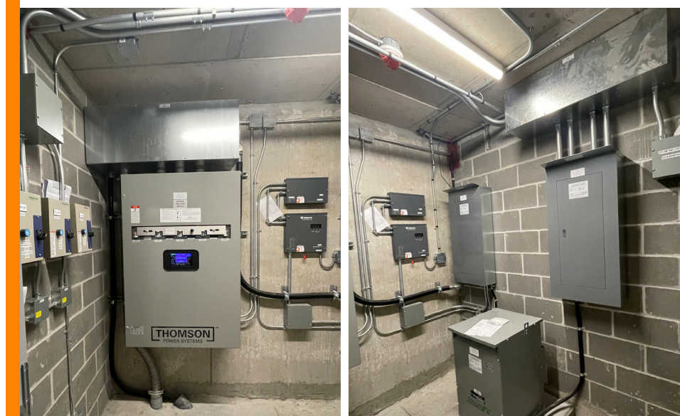
Electrical room with metering cabinets (Credit: Integral Group)
