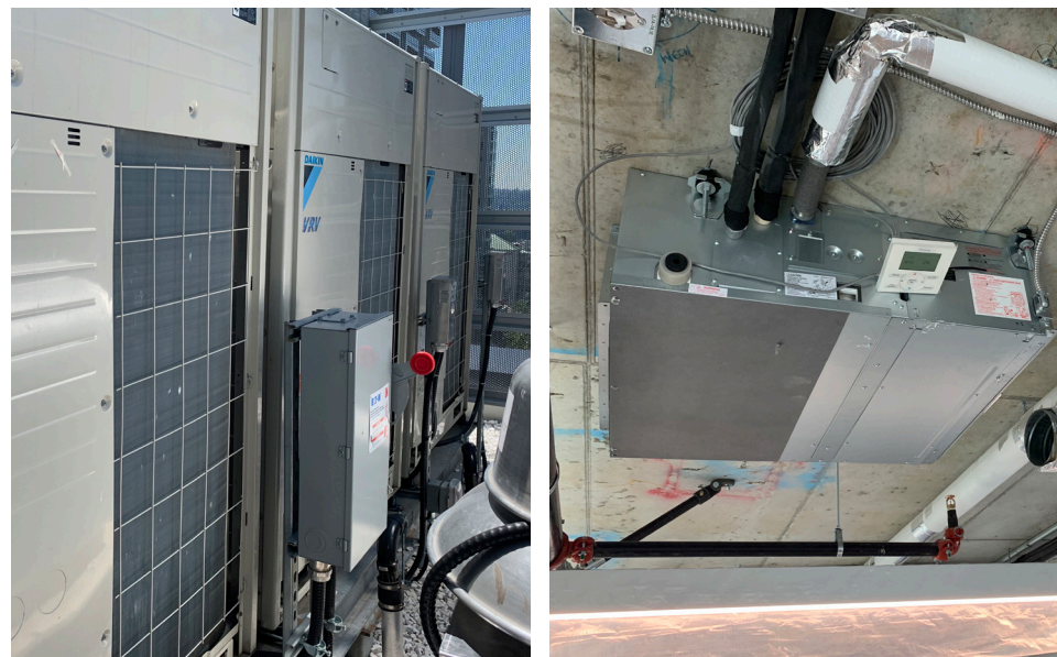
Left: Daikin condensing units; Right: Typical fan coil unit
